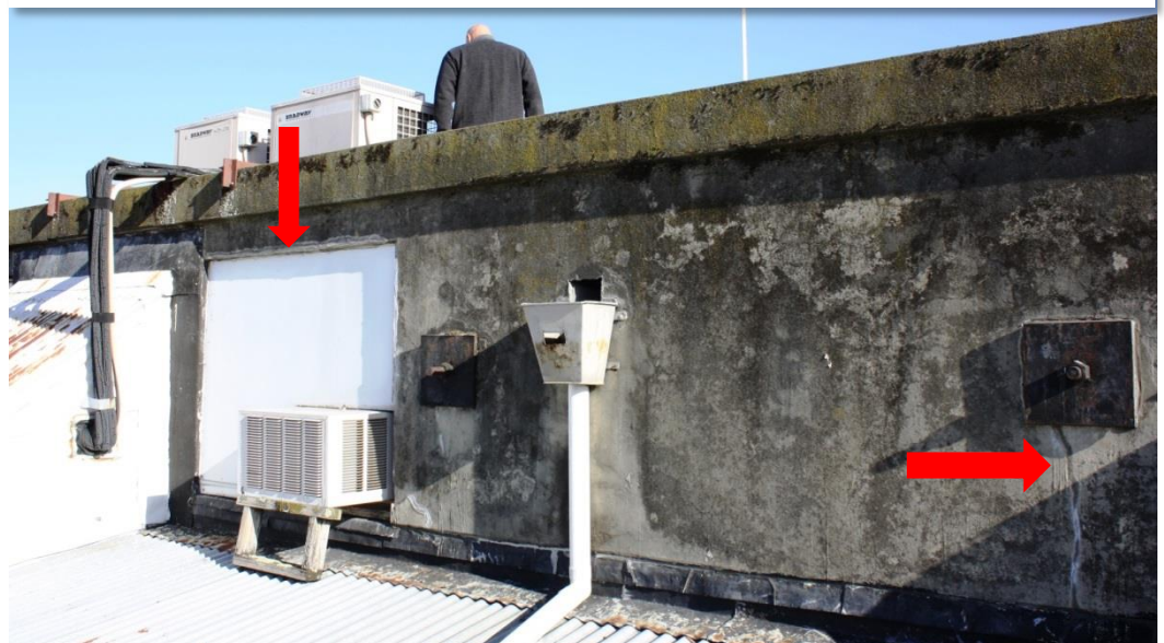
The top of the concrete wall that spans between the 1 st & 2 nd floor and covers the width of the building. This is the wall that holds back the façade – note the piece cut out and the cracks around the tie back bolts
