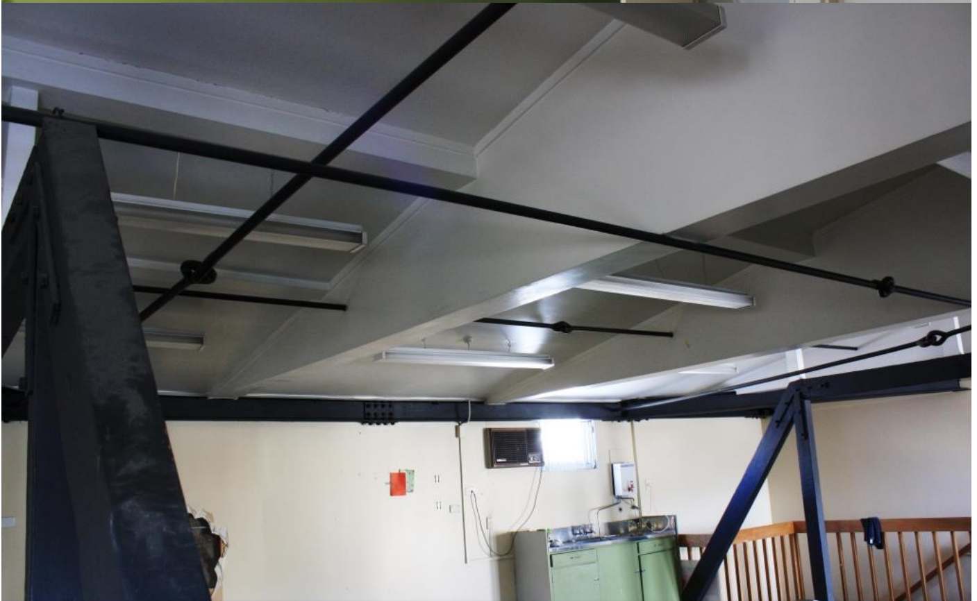
Above: Strengthening on the 3rd level, (2nd floor) after the Murchison earthquake with RSJ beams and metal ties between the façade and the interior concrete wall make the space practically unusable
