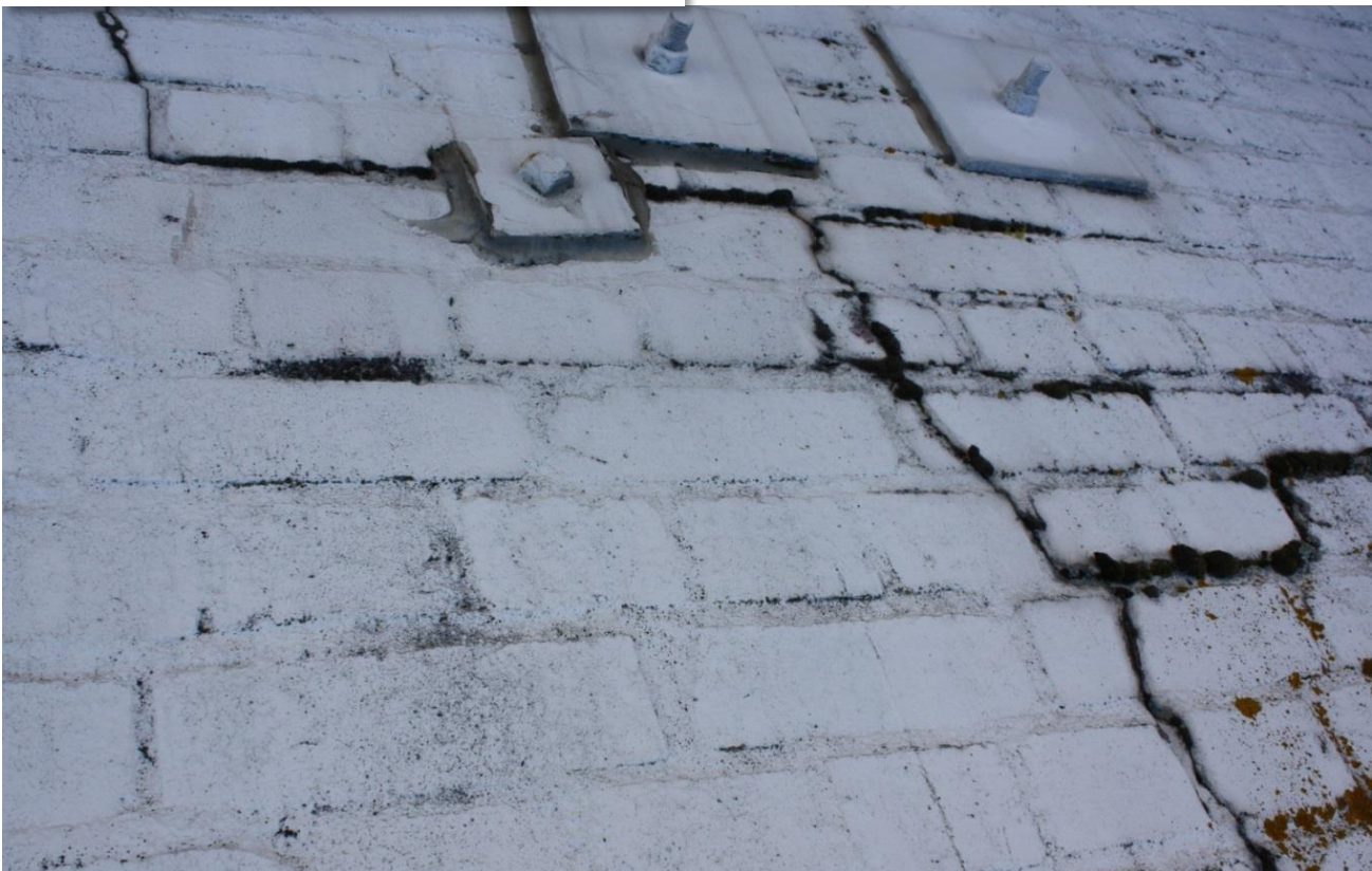
South facing boundary wall, above the party wall with the 'Pascoe's' building. Large cracks from the Inangahua earthquake, repaired with bolts & plates
