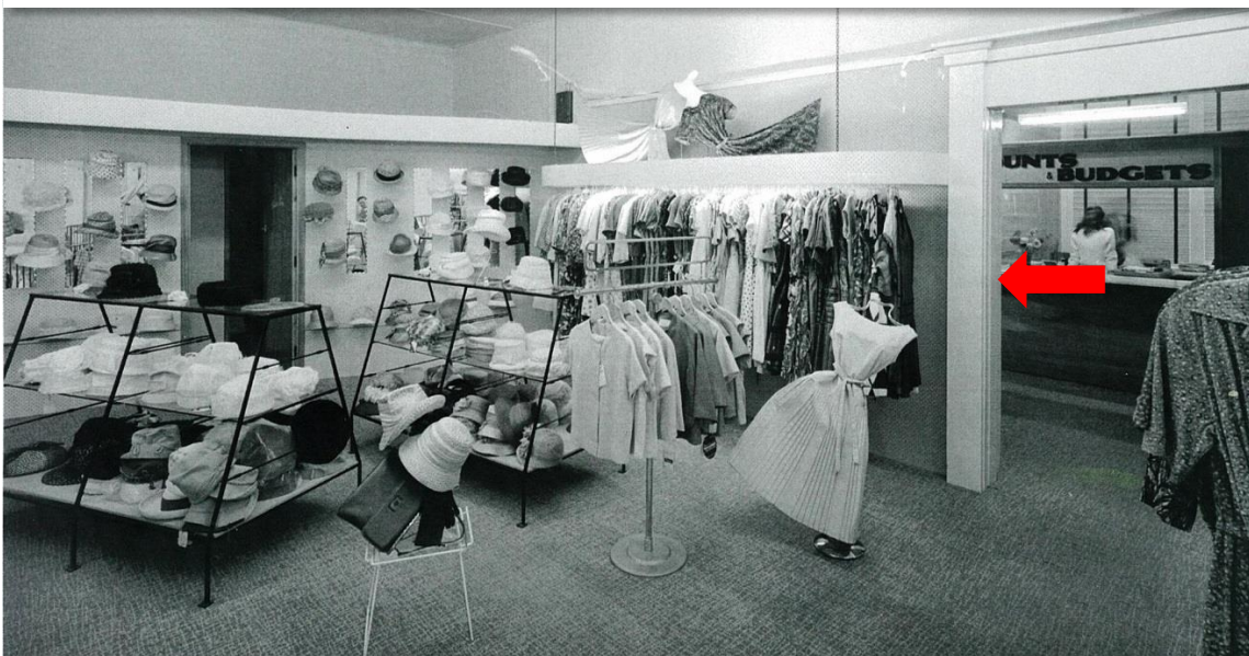
Hats & ladies fashions were on the second floor with the office visible through the archway towards the front of the building. Red arrow shows the suspended concrete wall that is tied to the façade of the building
