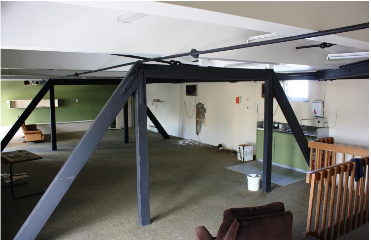
The 2 nd floor, (3 rd level), has the most compromised space
