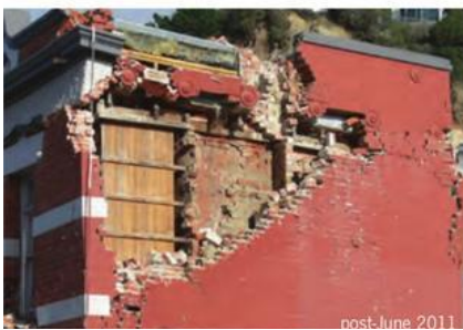
Above: Masonry falls outwards
