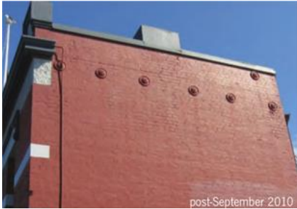
Unreinforced Masonry Building Post September 2010
