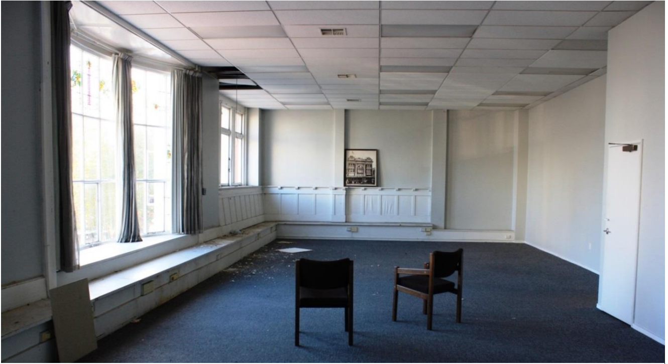
The 1 st floor , (2 nd level), is divided into two spaces by an internal concrete wall. The feature bay window that is so impressive from the outside of the building is divided over 3 floors. The middle third of the window is the only portion visible on the interior of the building. This was the old tea room space.
